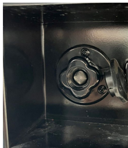
Figure 9-11: City Water Fill Port
