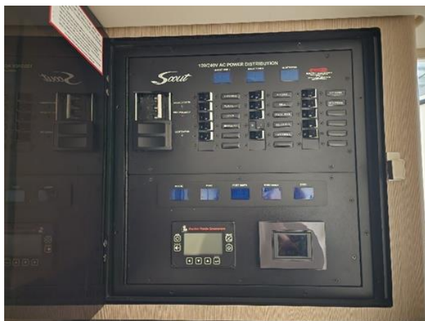
AC Main Distribution Panel
