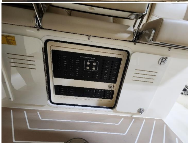
Battery Select Panel and AC/DC Panel
