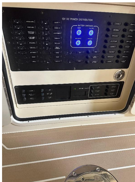
"Rocker" Style Circuit Breaker and push to reset breakers
