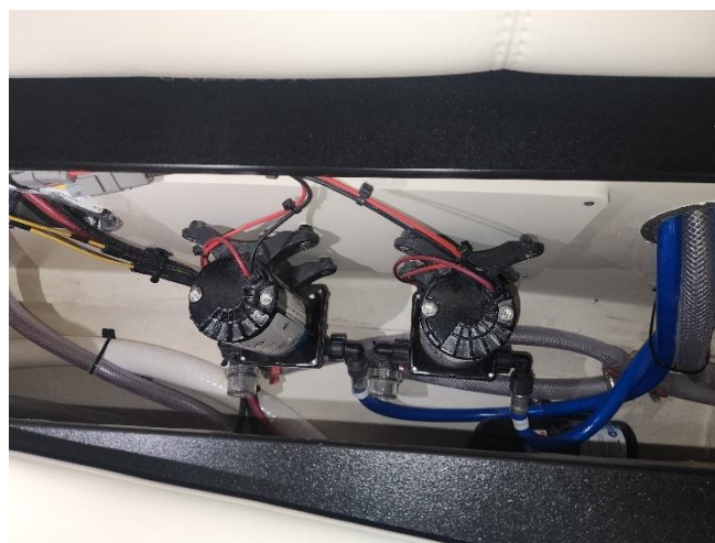
Fresh Water Pumps
