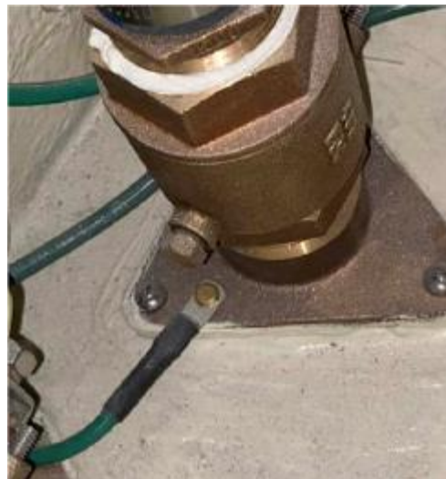
Thru-Hull Valve Bonding Wires & Connection
