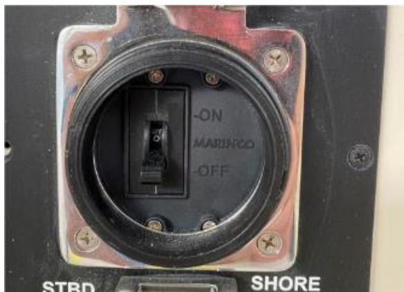
Shore Power Inlet Circuit Breaker
