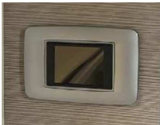
Air Conditioning Controller
