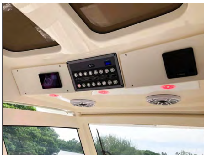
Typical Switch Panel In Hardtop
