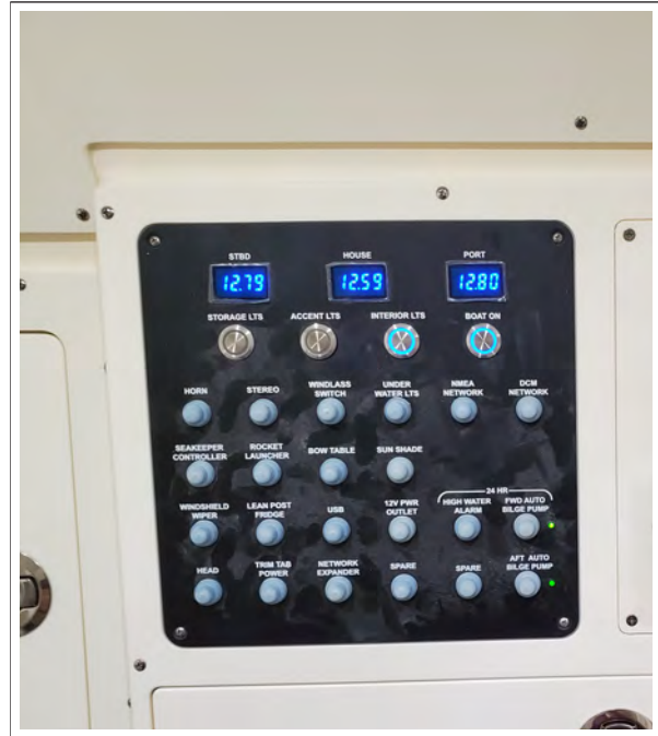
Cabin DC Panel Remote Battery Switches
