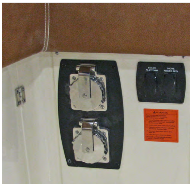
Shore Power Inlet Breaker & ELCI Inlet Panels
