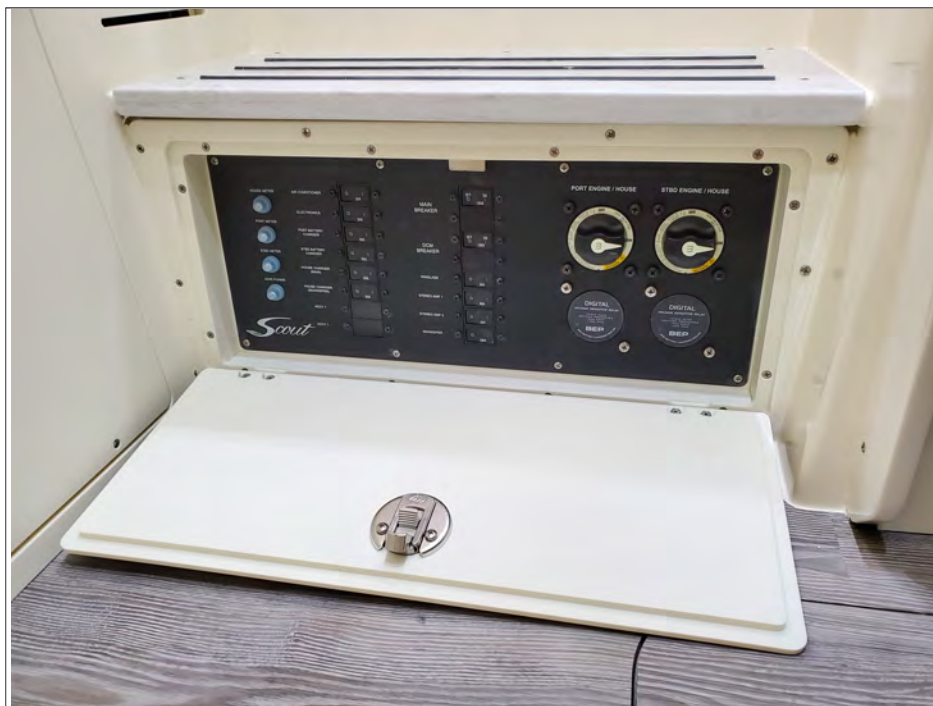
Cabin DC Breaker Panel
