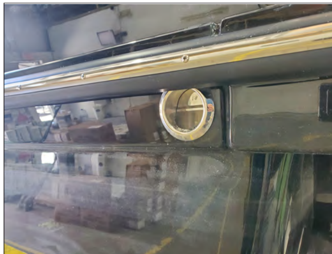
Scupper Drain Thru-Hull Fittings & Check Valves
