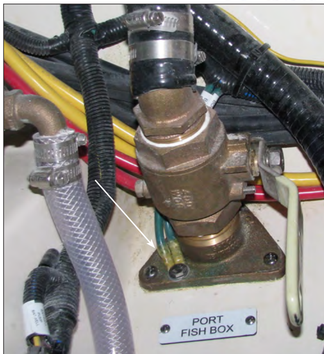
Thru-Hull Valve Bonding Wires & Connection
