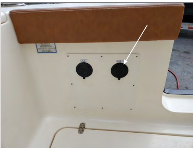
Fresh Water Washdown
