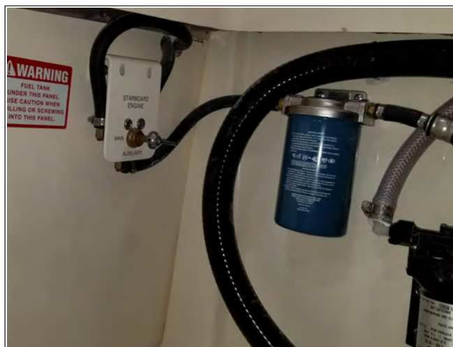
Dual Engine Starboard Fuel Filter & Stbd Engine Valve Manifold
