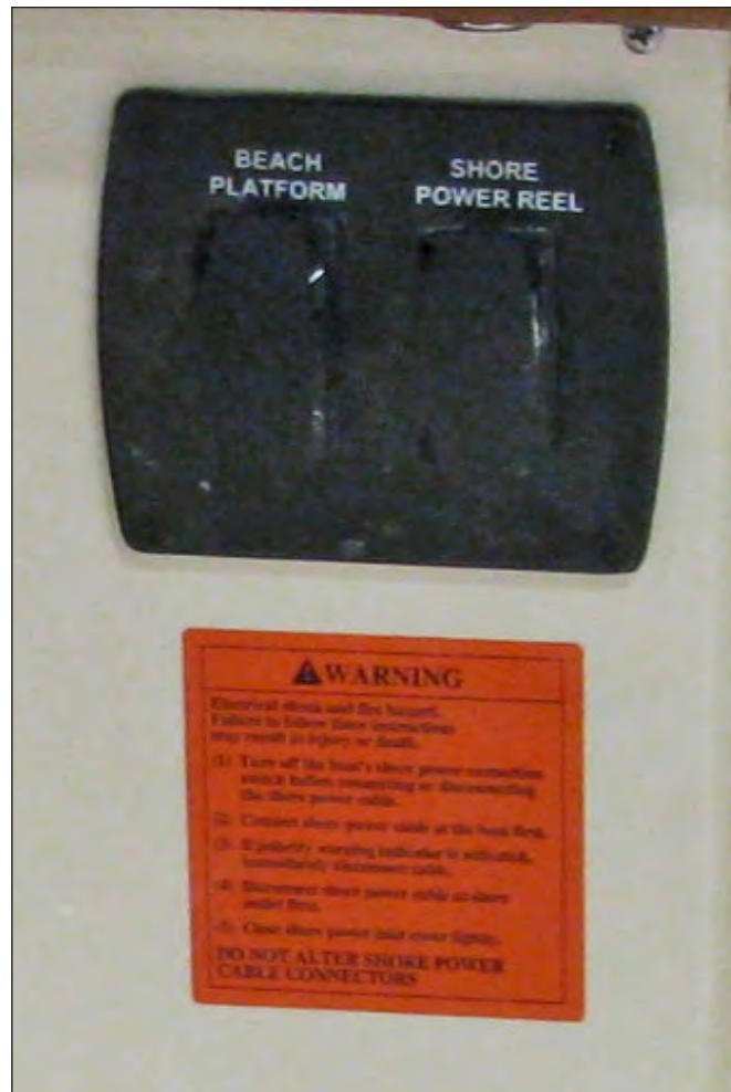
Shore Power Reel Switch
