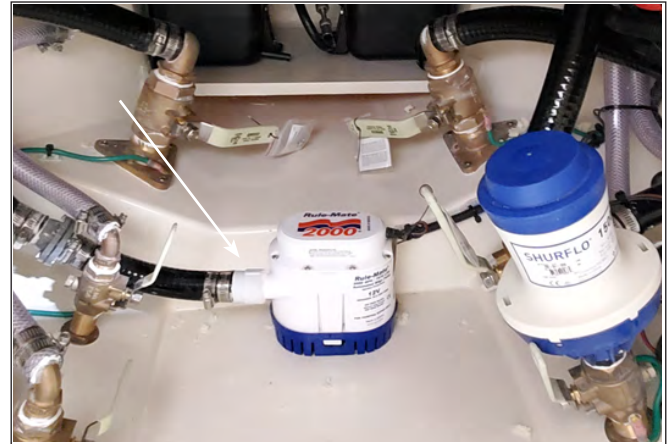
Aft Bilge Pump With Automatic Switch
