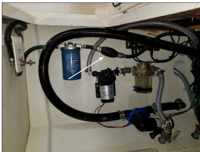
Fuel Primer Bulbs In Aft of Filters
