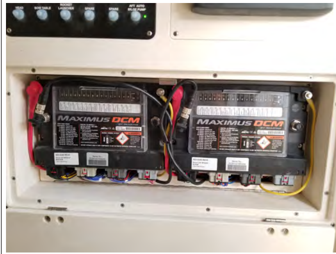
Electrical Systems Room Behind Steering Wheel
