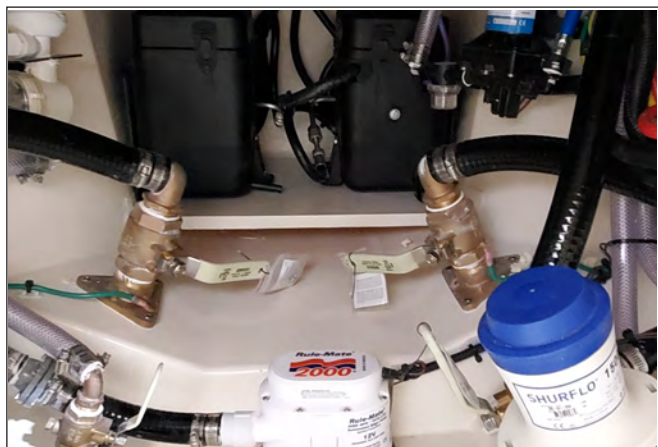
Port & Starboard Fishbox Pump Out Thru-Hull Fitting & Valve
