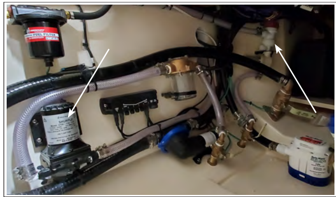
Typical Optional Air Conditioner and Optional SeaKeeper Cooling Pump
