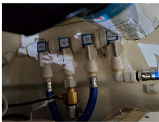
Fresh Water Pump Access Panel In Lower Aft Console
