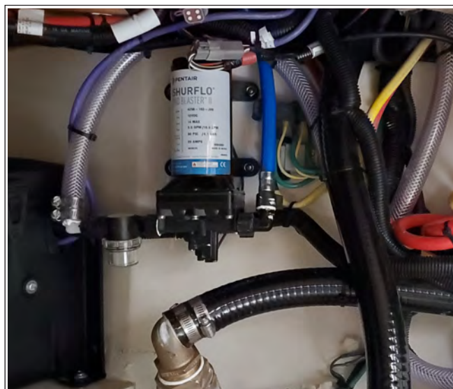
Raw Water Washdown Pump
