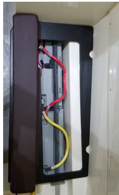
Engine Batteries Underneath Starboard Cushion & House Batteries are Underneath Port Cushion in the Console
