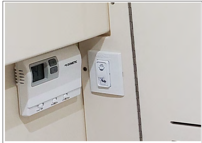
Typical Marine Head Control & AC Controller
