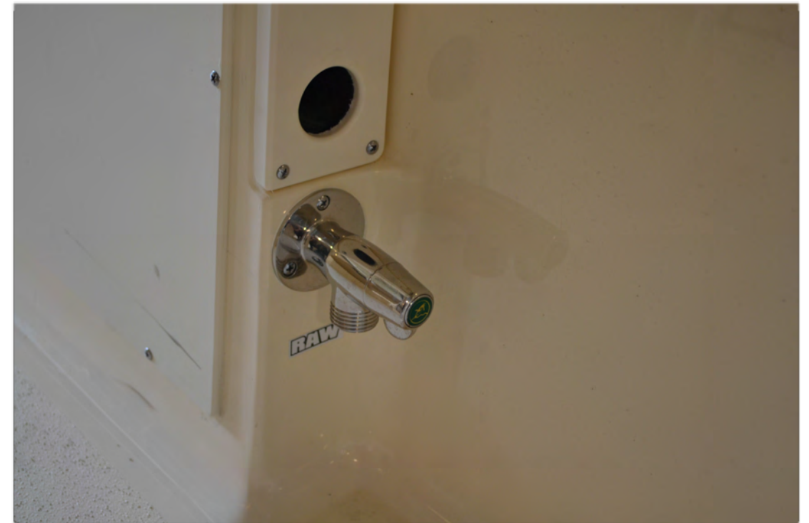
Raw Water Outlet
