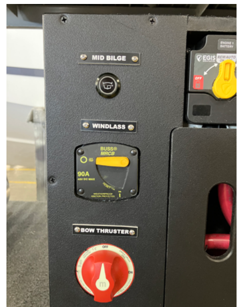
Bow thruster power switch
