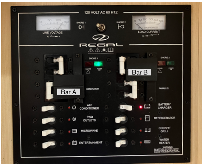
Main Distribution Panel (MDP)
