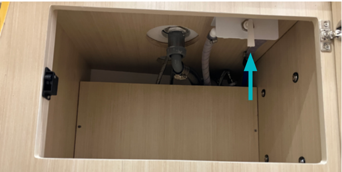
Shore water shutoff valve
