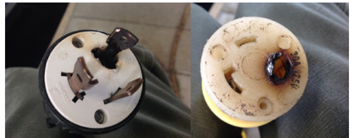
Examples of damaged shore power cords
