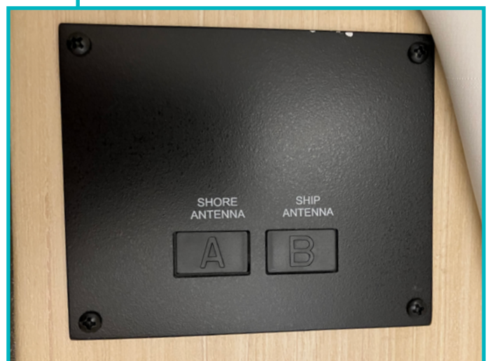
Coaxial splitter panel
