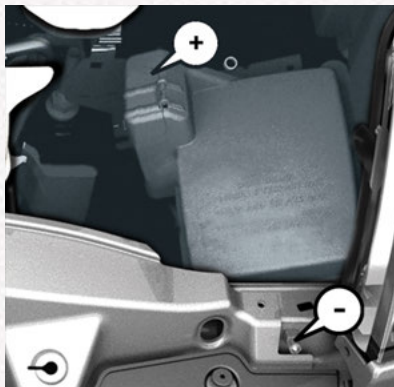
Remote Battery Posts
