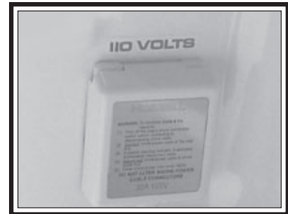
Shore Power Inlet
