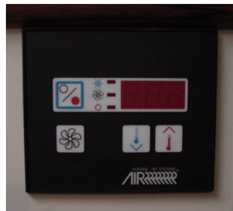
Air Conditioning Control Panel
