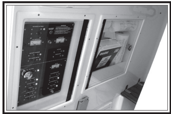
Electrical Panel and Towel Rack
