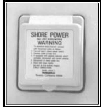
Shore Power Inlet
