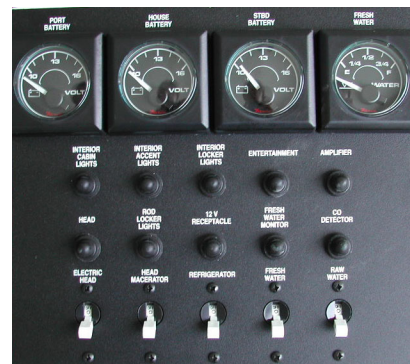
Cabin DC Breaker Panel
