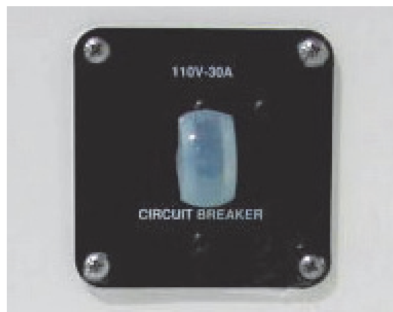
Shore Power Breaker
