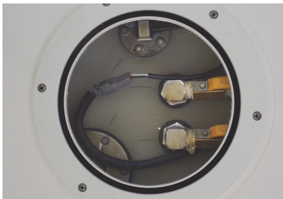
Gas Tank Valves
