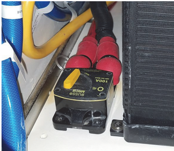
Main Battery Disconnect
