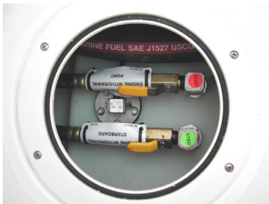
Fuel Valves Forward Tank
