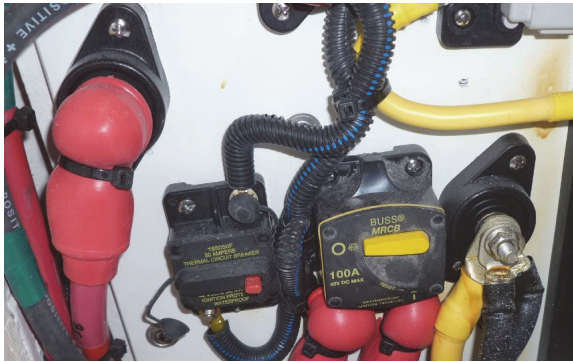
Main Battery Disconnect
