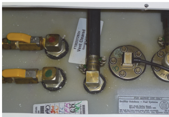
Gas Tank Valves
