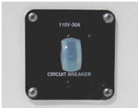
Shore Power Breaker
