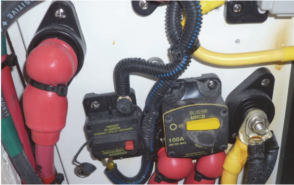
Main Battery Disconnect
