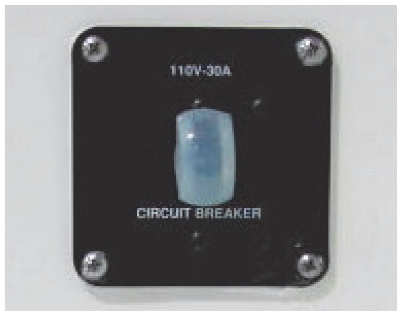
Shore Power Breaker
