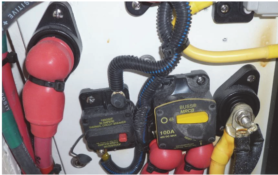
Main Battery Disconnect
