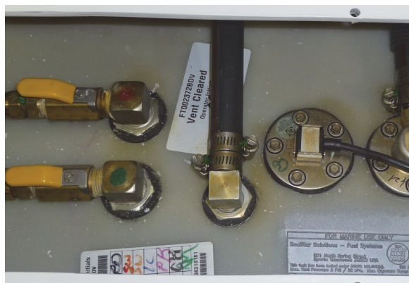
Gas Tank Valves
