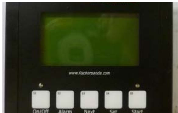
Generator control panel
