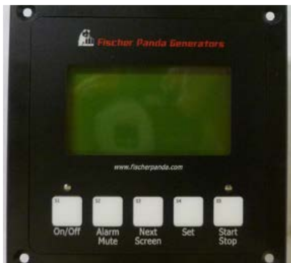
Generator control panel on the AC MDP
