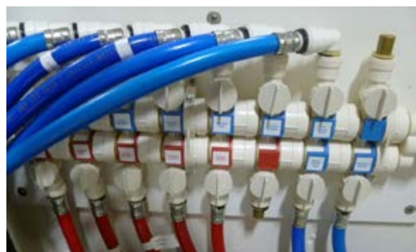
Water system manifold
