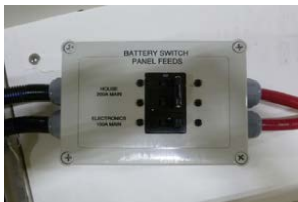
Battery switch panel feeds
