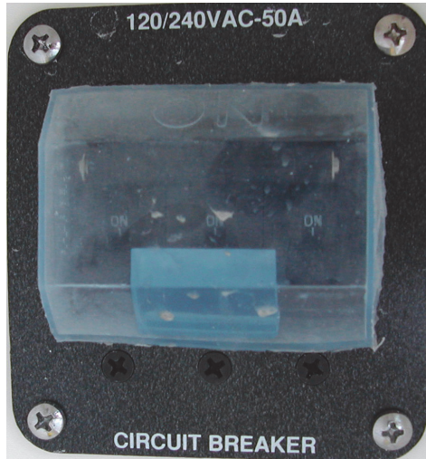
Shore Power Breaker
