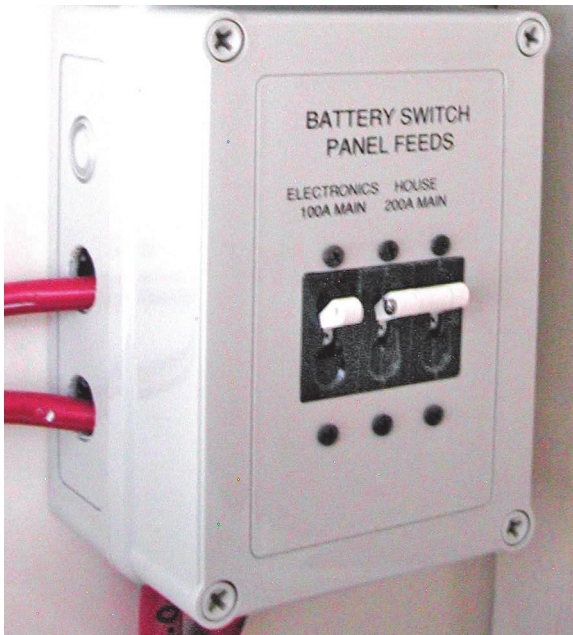
Battery Switch Panel Feeds
