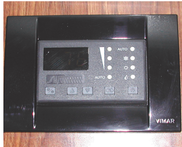
Air Conditioning Control Panel
