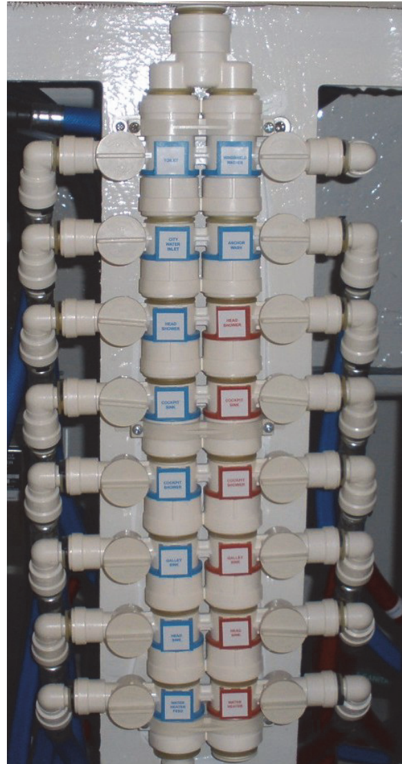
Water System Manifold (Typical)
