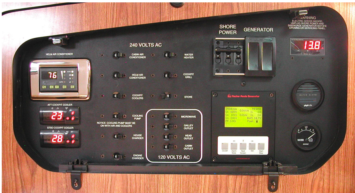
AC Main Distribution Panel (AC MDP)
