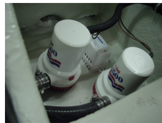
Aft Bilge Pumps (Typical)
