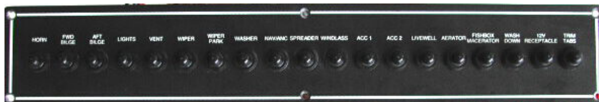
Helm Breaker Panel
