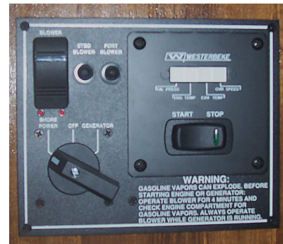
Gasoline Generator Panel
