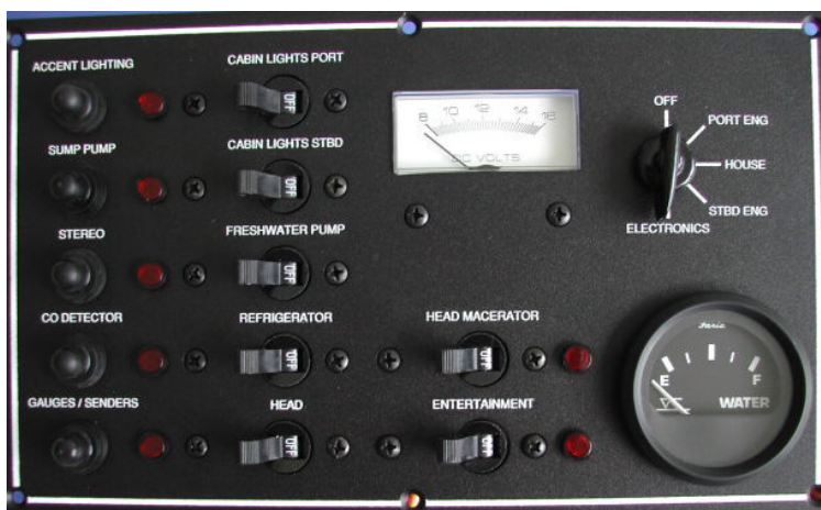
Cabin DC Breaker Panel (typical)
