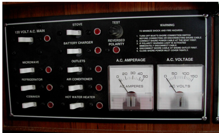
AC Breaker Panel
