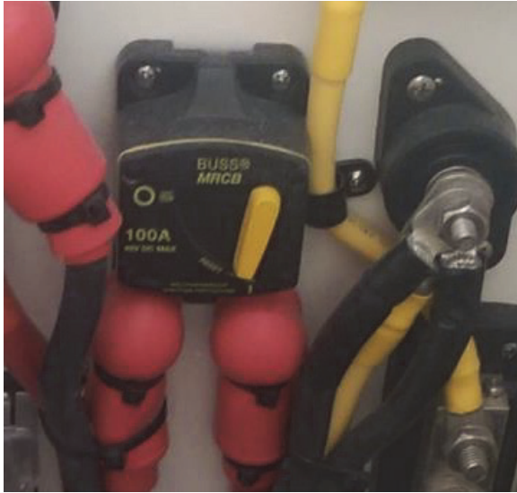
Main Electronics Battery Disconnect
