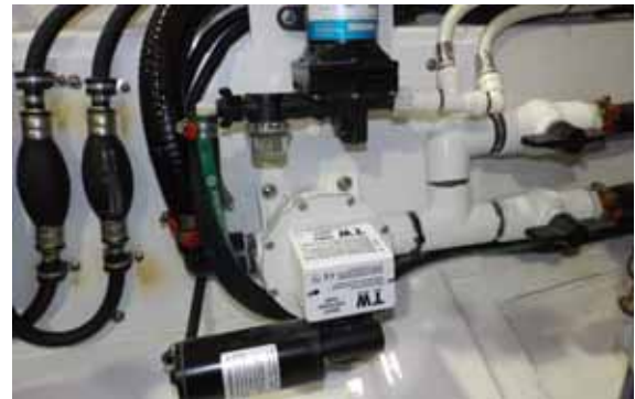
Fishbox Drain Manifold
