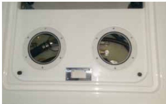
Gas Tank Valves
