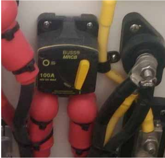
Main Electronics Battery Disconnect
