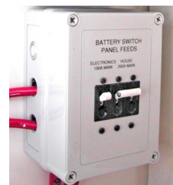
Battery Switch Panel Feeds
