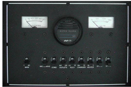
AC Breaker Panel
