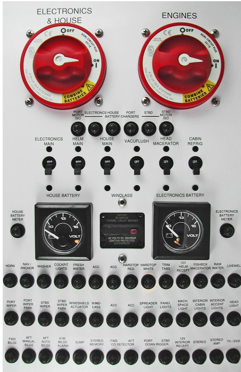
Main Distribution Panel (MDP)
