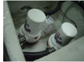
Bilge Pump (Typical)
