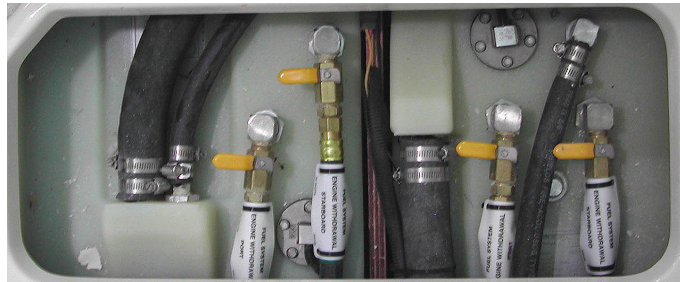
Fuel Tank and Valves
