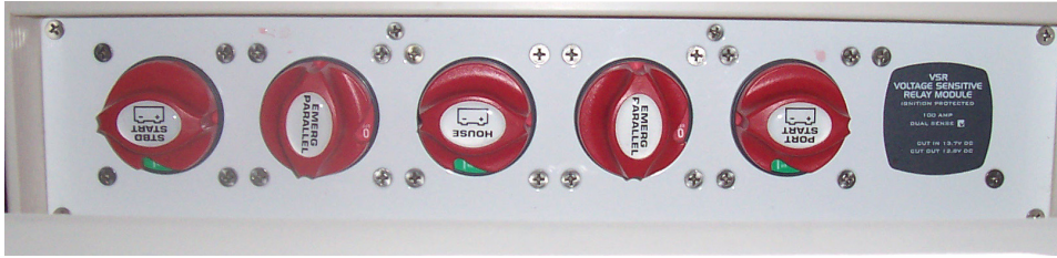
Battery Switch Panel
