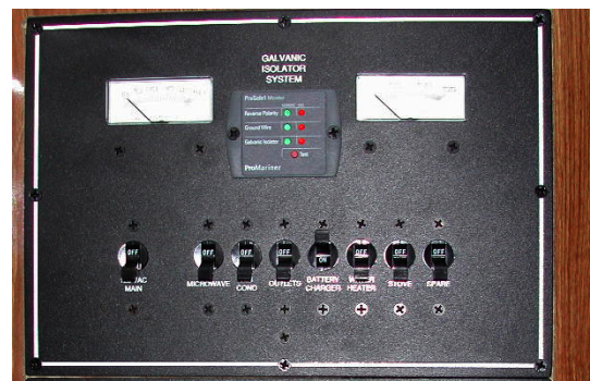
AC Breaker Panel
