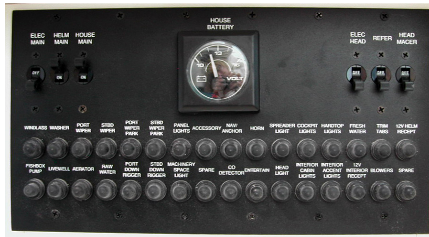
DC Main Distribution Panel (MDP)
