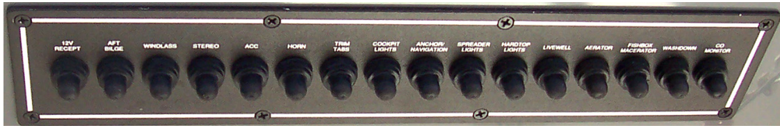
Helm Breaker Panel
