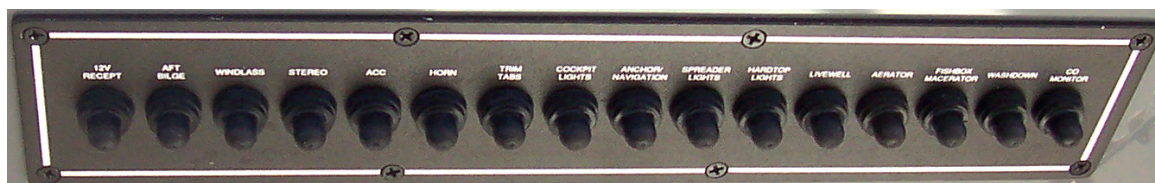
Main Distribution Panel (MDP)
