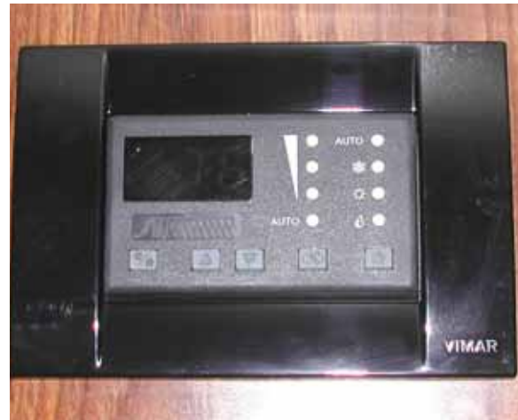
Air Conditioning Control Panel
