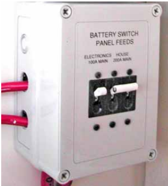
Battery Switch Panel Feeds
