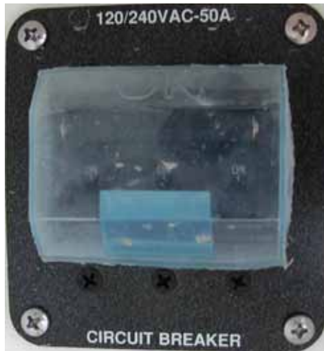
Shore Power Breaker
