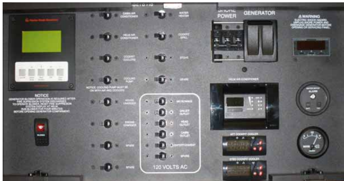
AC Main Distribution Panel (AC MDP)
