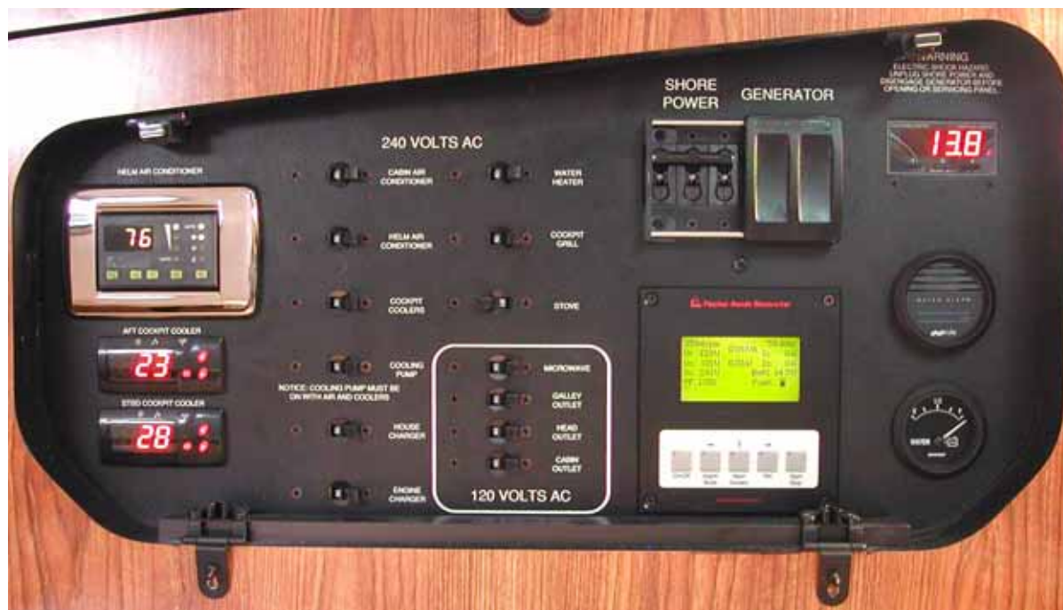
AC Main Distribution Panel (AC MDP)
