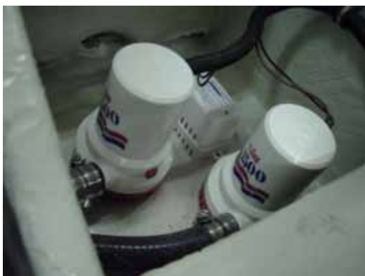
Aft Bilge Pumps (Typical)
