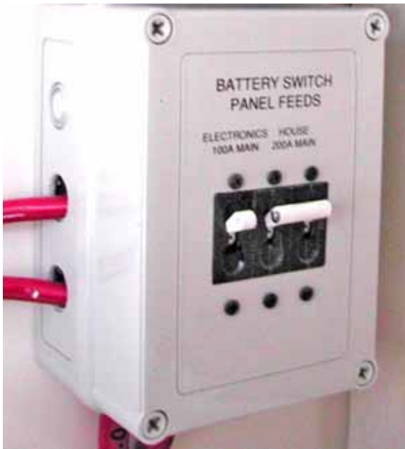
Battery Switch Panel Feeds
