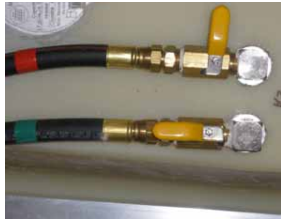
Fuel Tank Valve - Starboard
