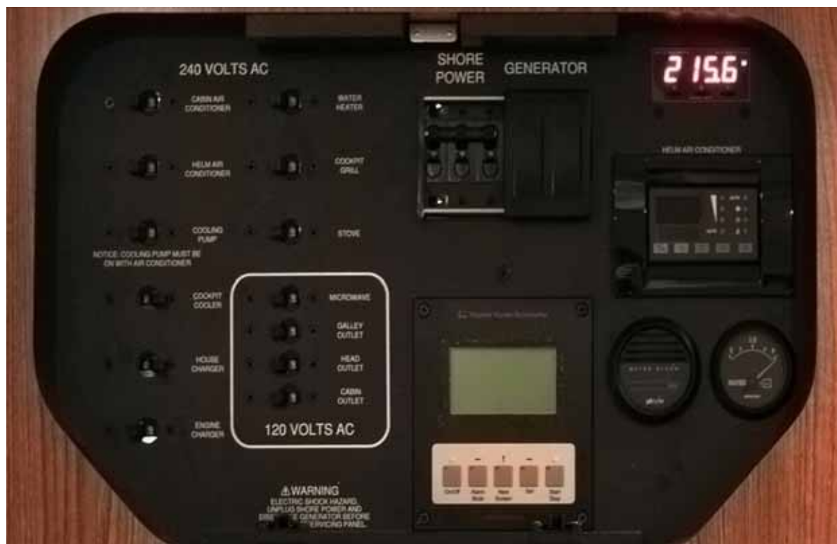
AC Main Distribution Panel (AC MDP)
