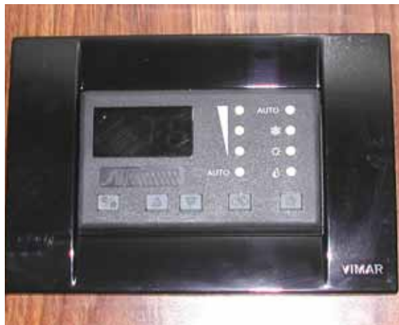
Air Conditioning Control Panel
