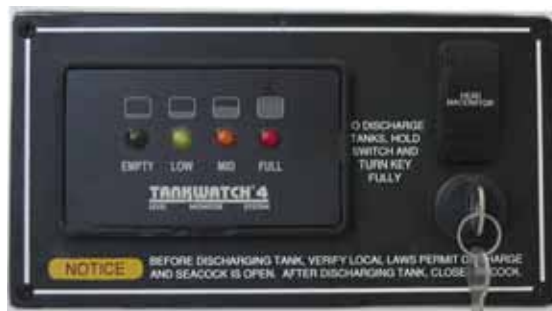
Head Switch Panel
