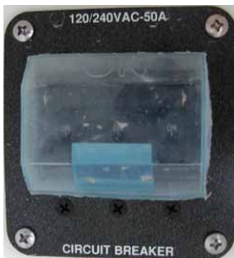
Shore Power Breaker
