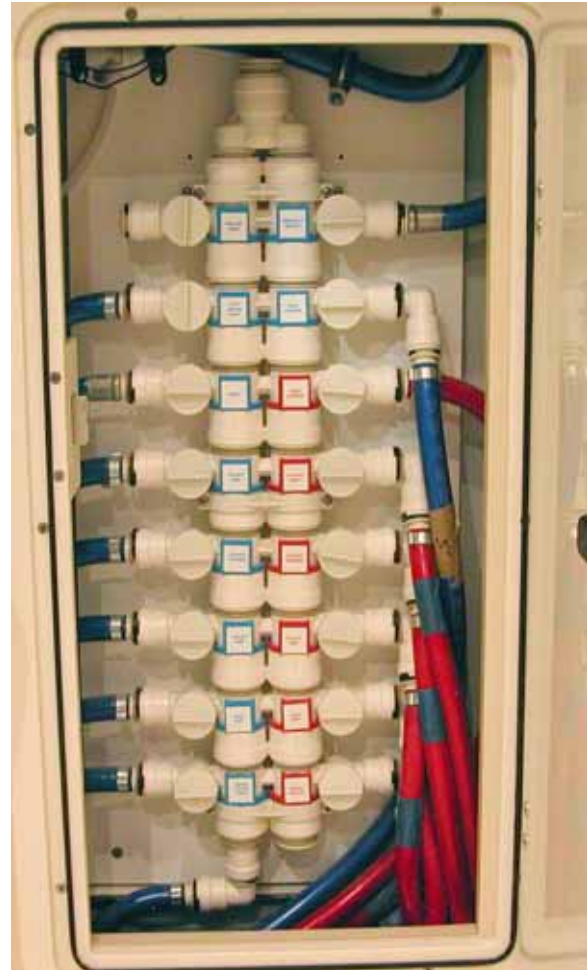
Water Shut-Off Valves
