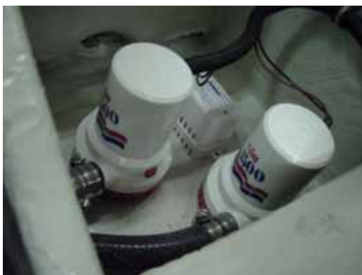
Aft Bilge Pumps (Typical)
