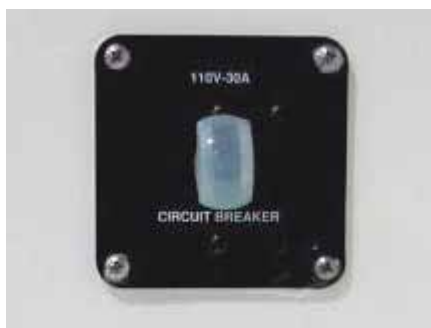
Shore Power Breaker
