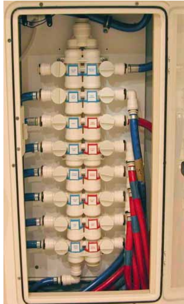
Water Shut-Off Valves
