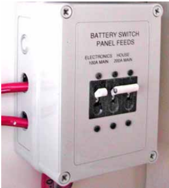
Battery Switch Panel Feeds
