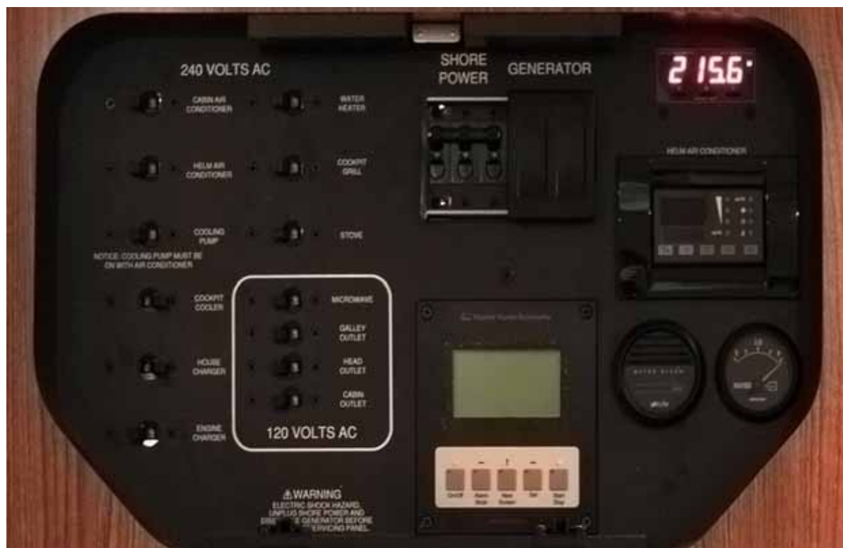
AC Main Distribution Panel (AC MDP)
