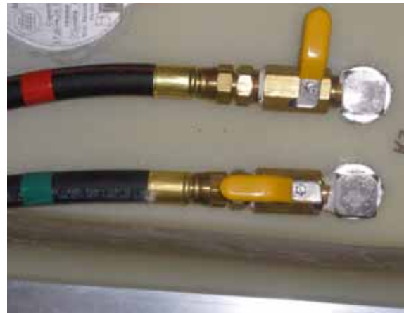
Fuel Tank Valve - Starboard
