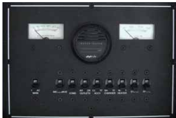
AC Breaker Panel
