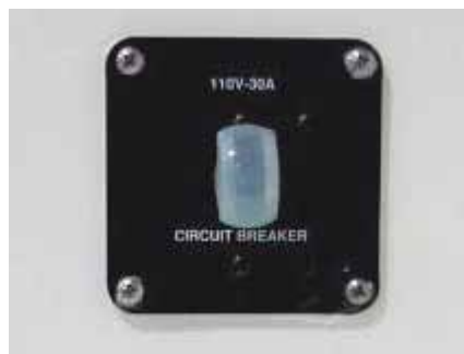
Shore Power Breaker
