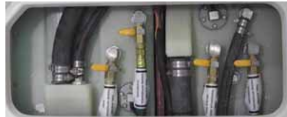
Fuel Tank Valves
