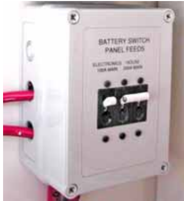
Battery Switch Panel Feeds
