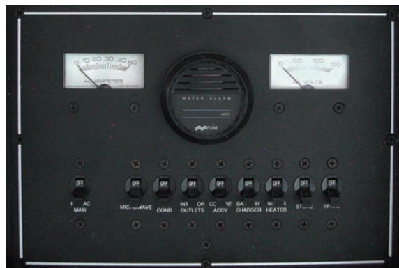
AC Breaker Panel
