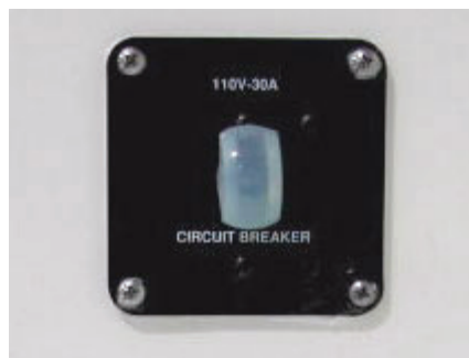
Shore Power Breaker
