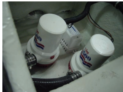
Bilge Pump (Typical)
