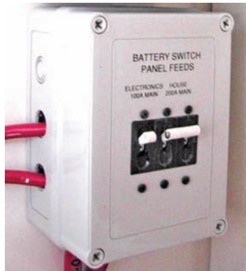
Battery Switch Panel Feeds
