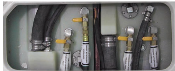
Fuel Tank and Valves
