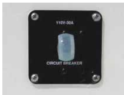
Shore Power Breaker
