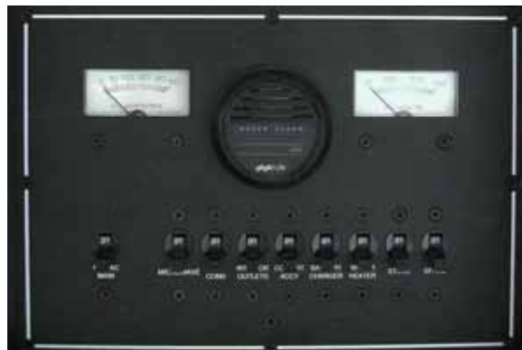
AC Breaker Panel
