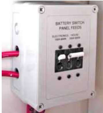
Battery Switch Panel Feeds
