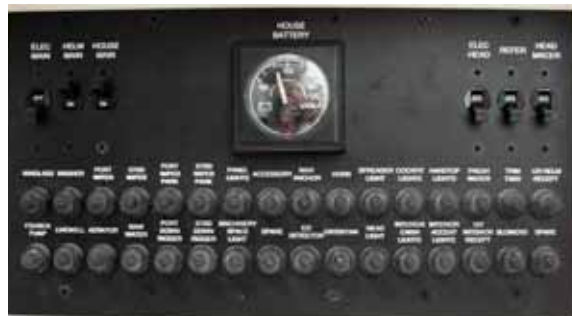
DC Main Distribution Panel (MDP)
