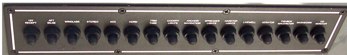
Main Distribution Panel (MDP)
