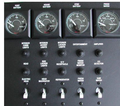
Cabin DC Breaker Panel
