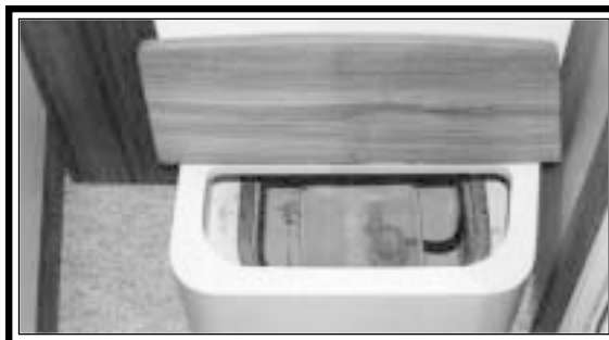
Shower and Cabin Drain Sump Pump
