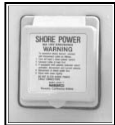
Shore Power Inlet
