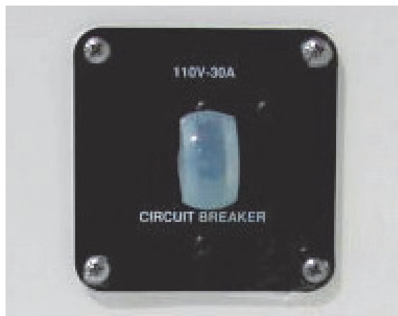
Shore Power Breaker
