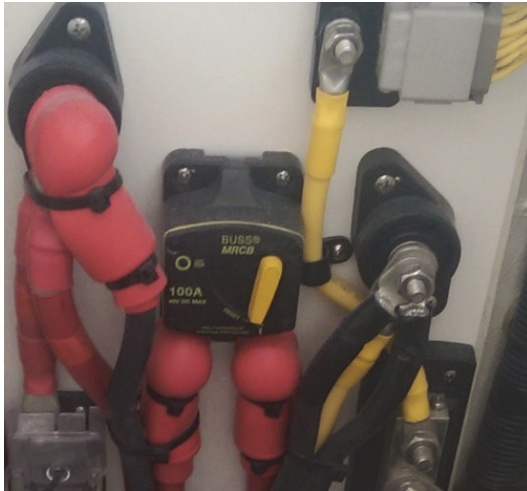
Main Battery Disconnect
