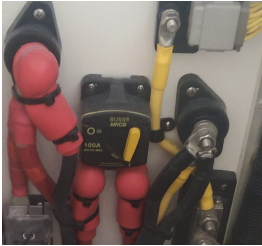
Main Battery Disconnect
