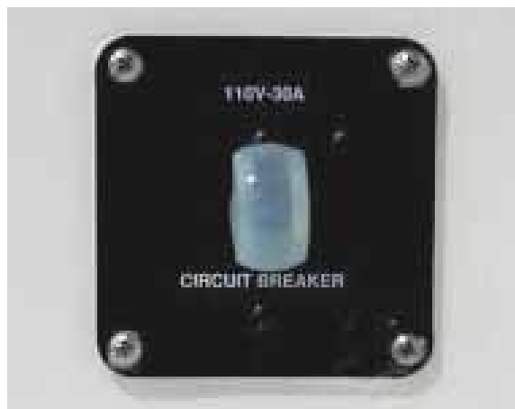
Shore Power Breaker
