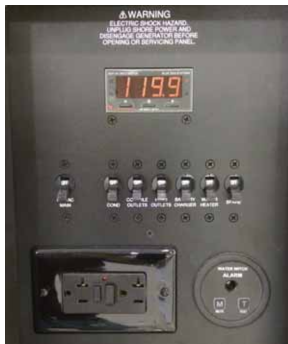
A.C. Distribution Panel
