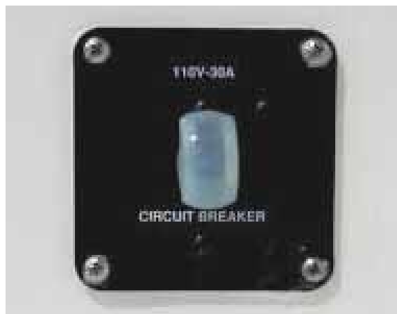
Shore Power Breaker
