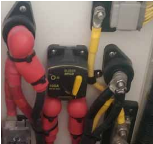
Main Battery Disconnect
