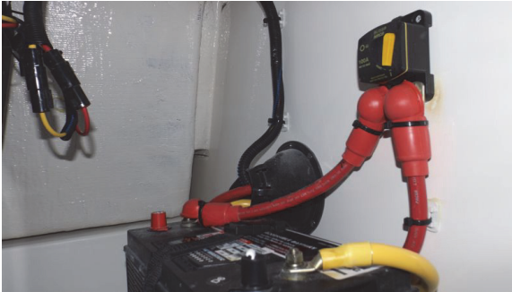
Main Battery Disconnect
