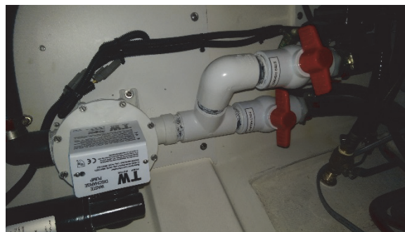
Fishbox Drain Valves
