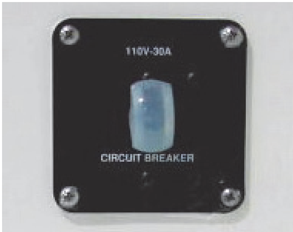
Shore Power Breaker
