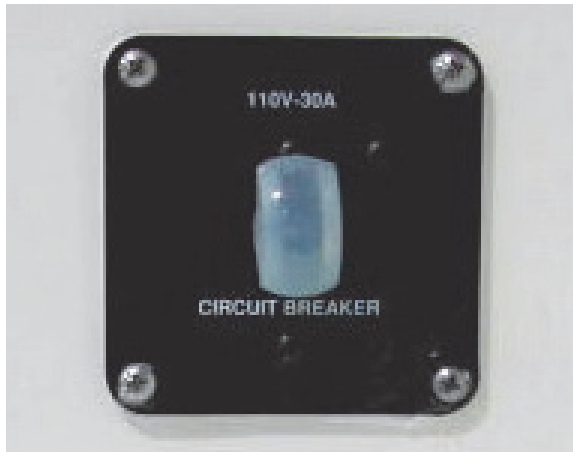
Shore Power Breaker
