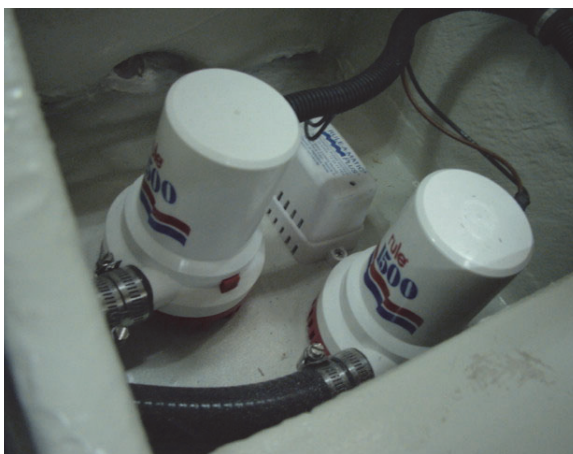
Bilge Pump (Typical)
