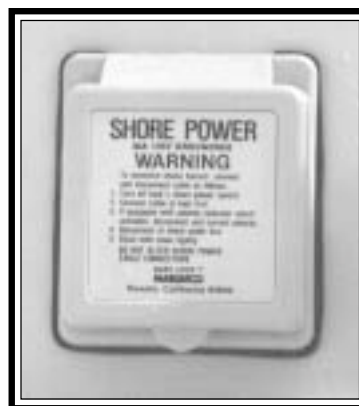
Shore Power Inlet
