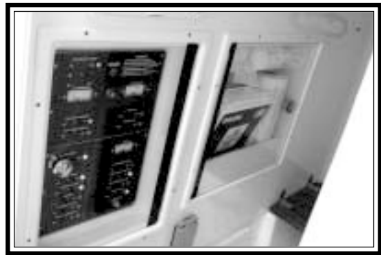
Electrical Panel and Towel Rack
