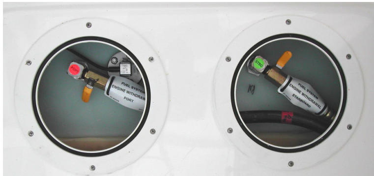
Fuel Valves Aft Tank
