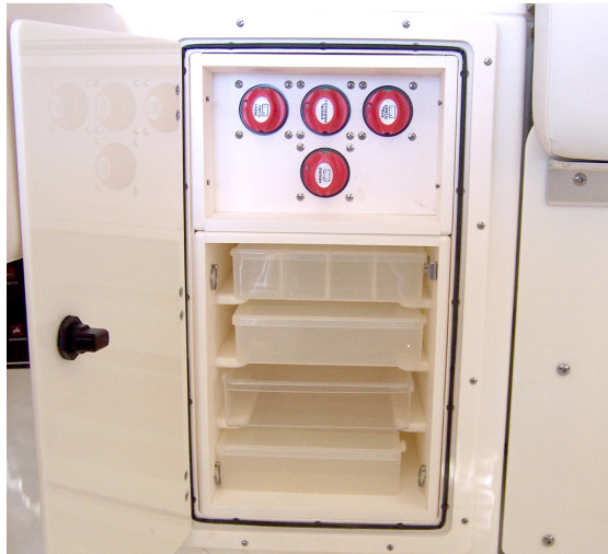
Battery Switch Panel
