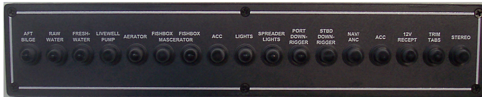
Main Distribution Panel
